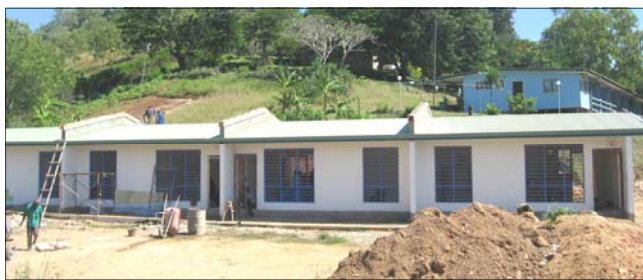
The new NRI staff flats comprising four, two-bedroom units are nearing completion.
