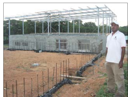
James Tongore, Site Manager for Heduru Contractors, stands next to the site that will become the new headquarters for the IT, Library, Production, and Publishing Division, next to the new Administration offices.
